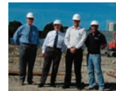
Pictured above on the Southern Cross University Building 'A' Site are, from left to right, Southern Cross University - Prof. Bryan Rothwell, Vice Chancellor, Prof. Paul Clark, Glenzeil - Brian Gabriel, Gerrod Williams
